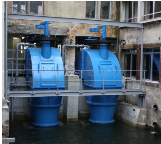
Photo 2. The two Siphon turbines set at Vallorbe, designed with MHyLab's hydraulic profile (2.5 m 3 /s per machine, 2.1 m head, total electrical output: 85 kW, external runner diameter: 1.25 m) (©MHyLab)
